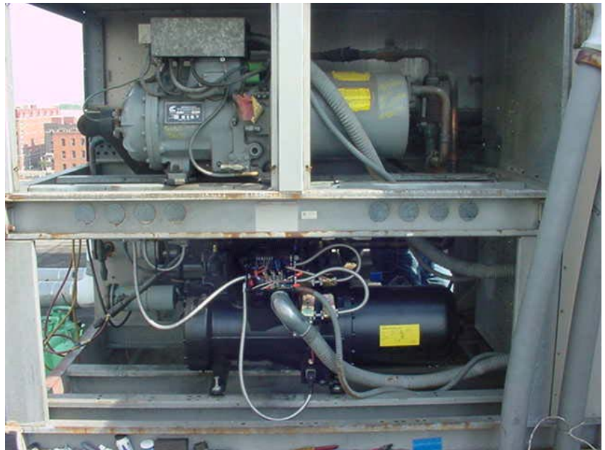
Old installation on top — new compressor below.
